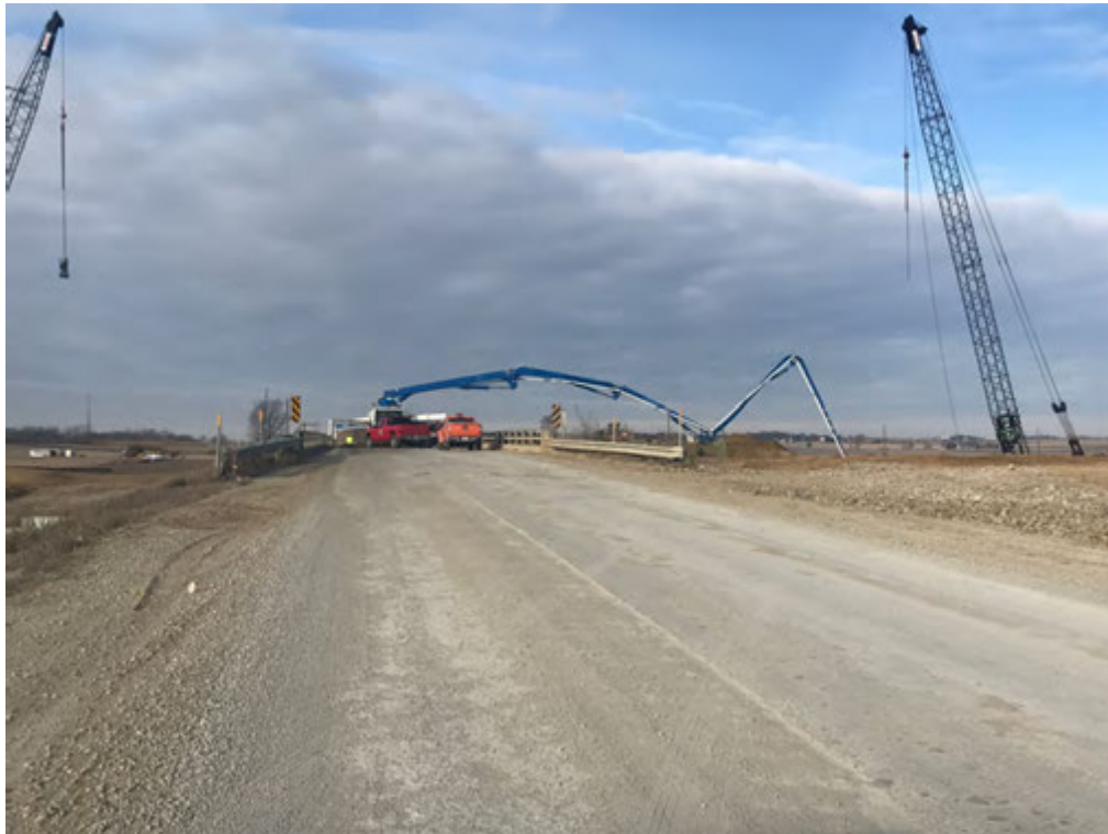
Closing of Forevergreen Rd for contractors to pump concrete for new bridge footings
