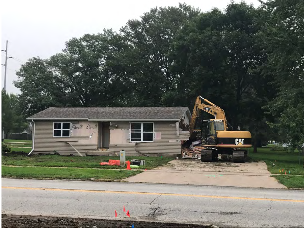
Demolition of 1 of the 3 houses at the Penn and Front St intersection
