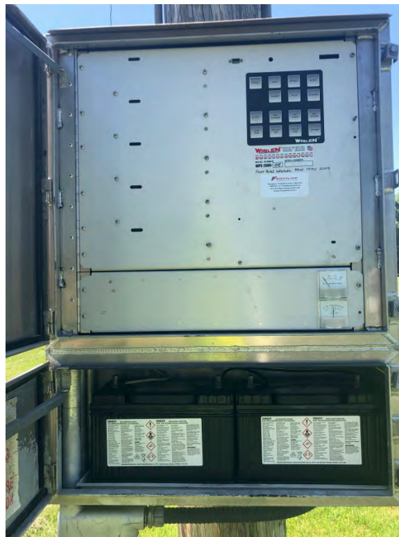
Warning Siren Cabinet. Heavy Duty batteries at bottom power sirens to eliminate power outage failure
