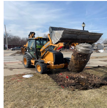
Park Staff removing the Old clock footing in preparation Dubuque St. Phase 1
