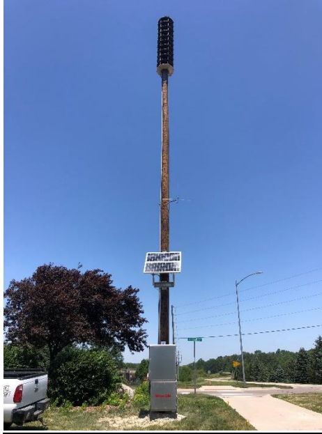
Scales Bend Rd/Pheasant Dr new siren installed
