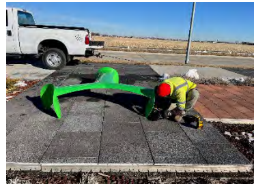
Tri-bench vandalism repair at the Centennial Park Parklet.
