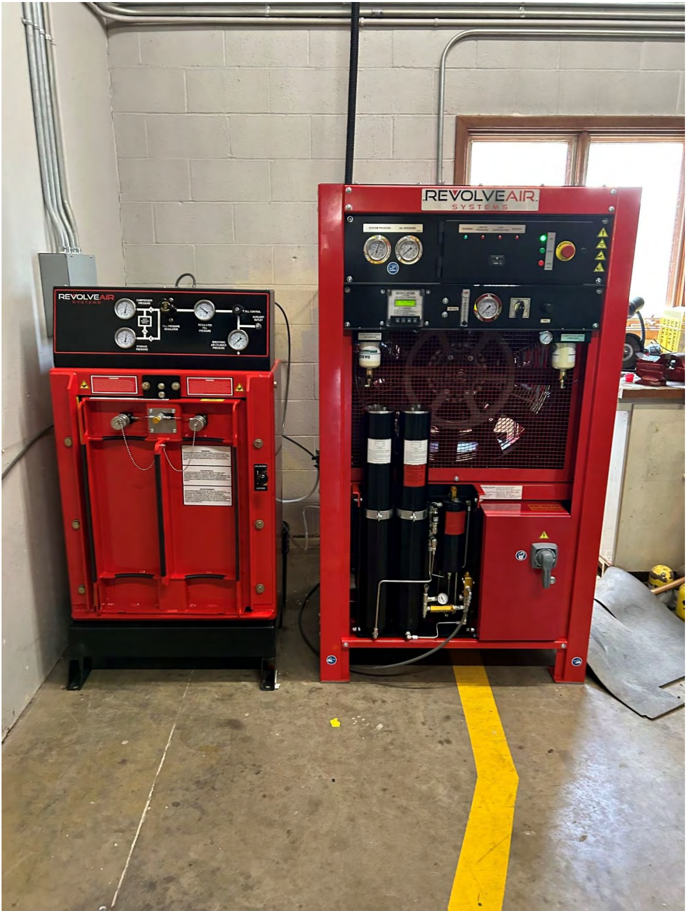
New Revolve Air compressor and fill station.
