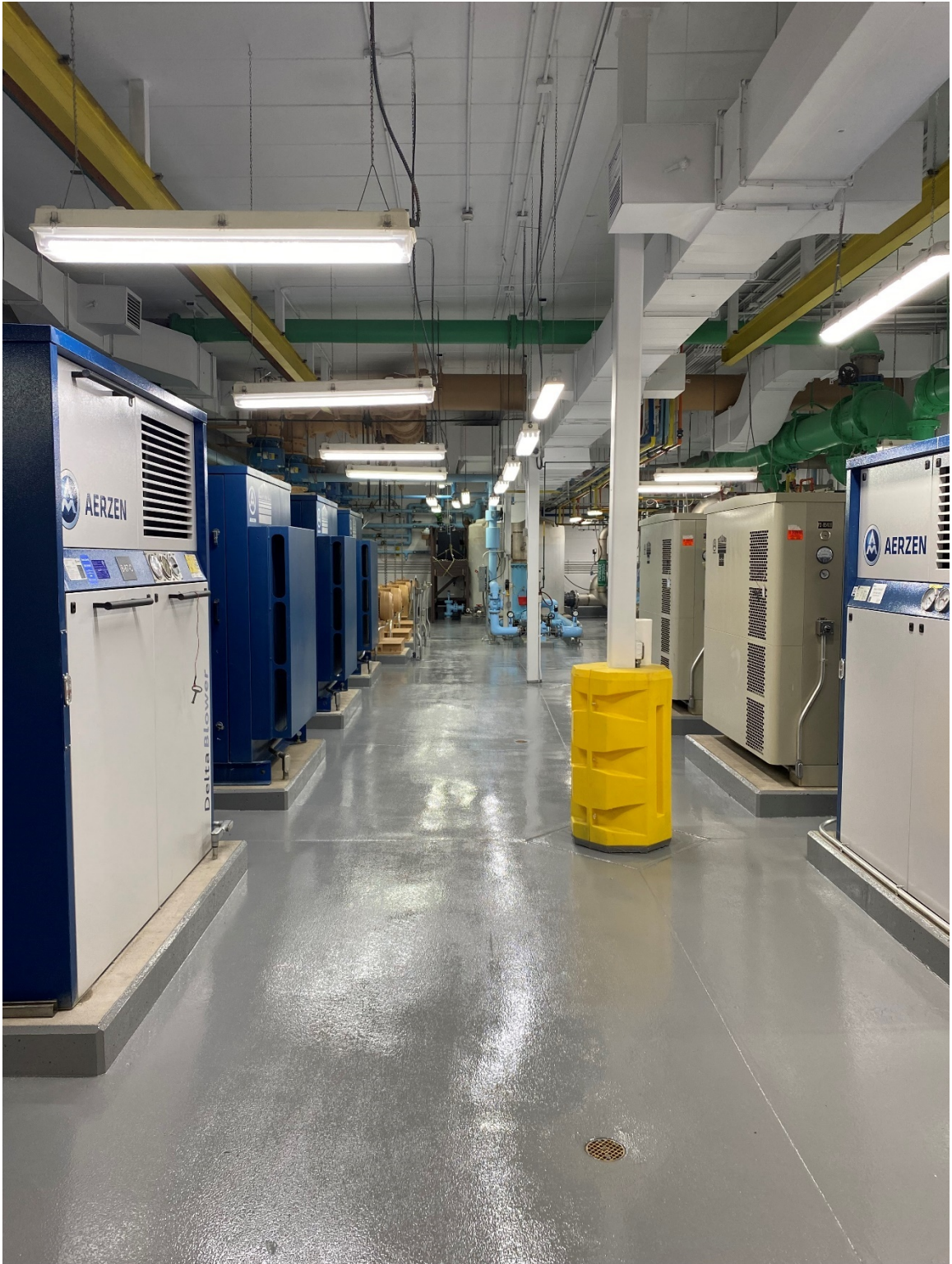
Painted Floor and Equipment
