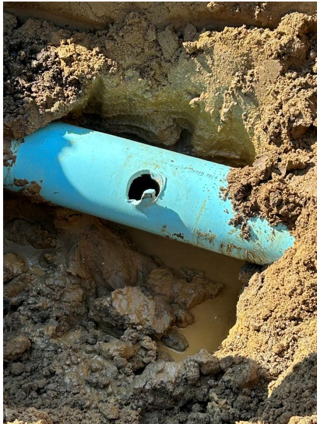
Centro Way force sewer damage
