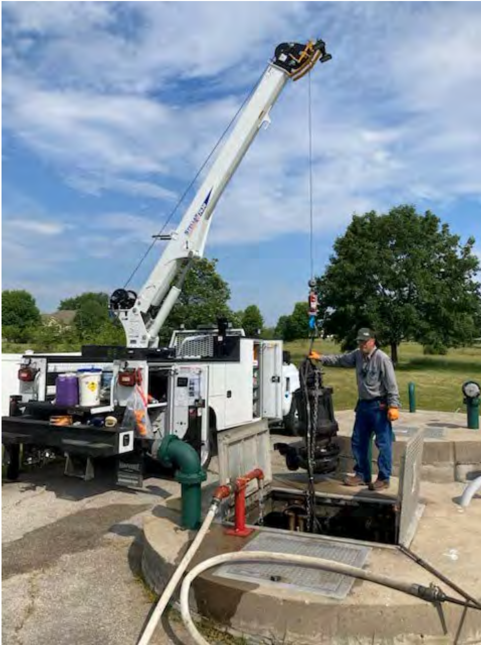
Cedar Springs Lift Station – Pump pulled and Inspected – Volute Casing Repairs Made
