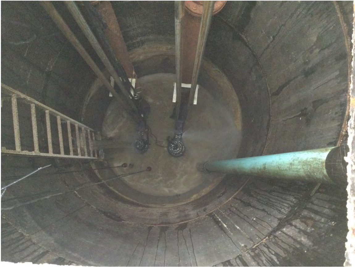
Progress Park Lift Station - pump discharge blow-by
