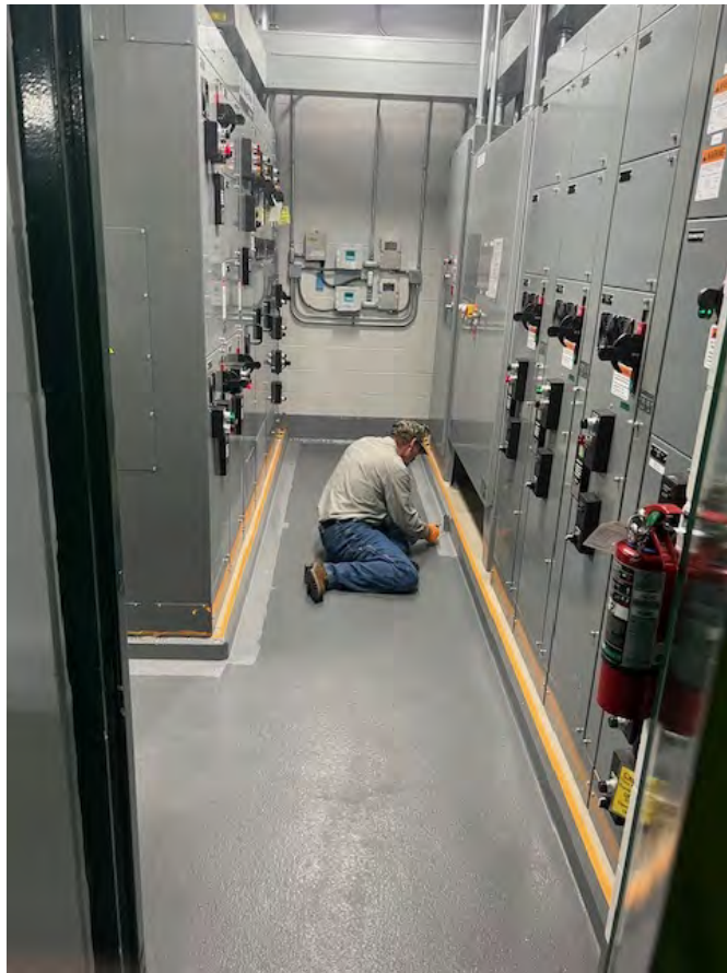
MBR (phase1) MCC Room
