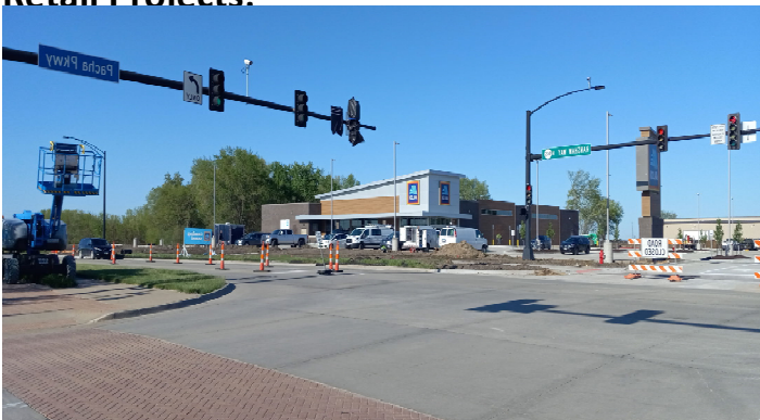
Crews are nearing completion of Aldi Food Store Grand opening is scheduled for May 2
