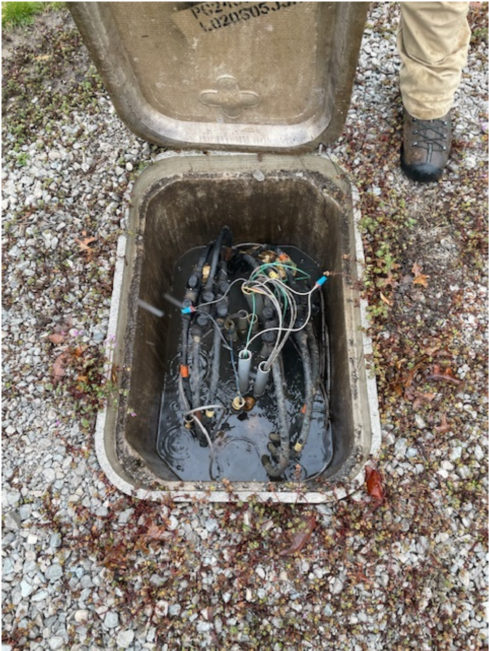
EQ Conduit Handhole filled with water
