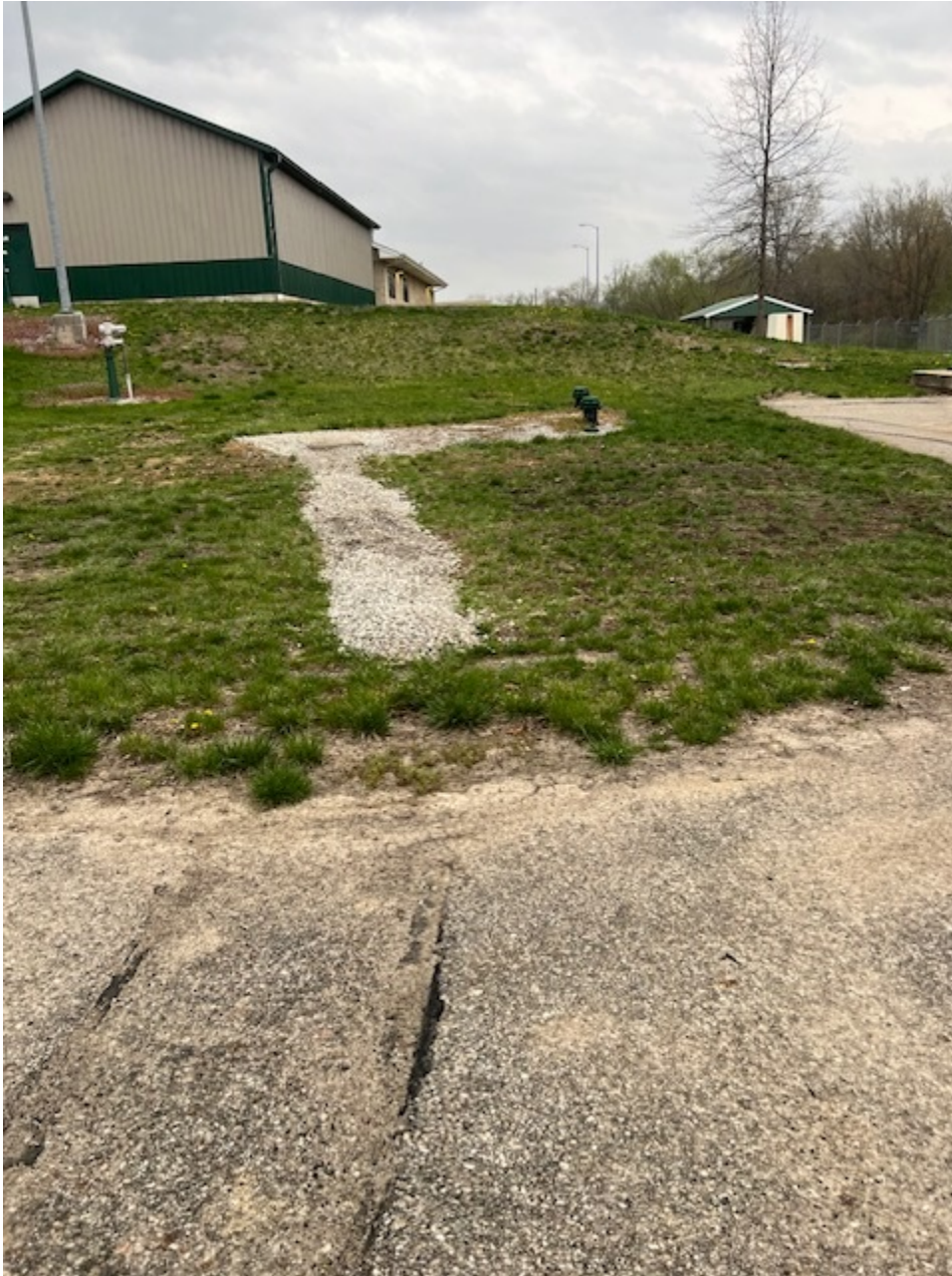
Drainage rock installed with tile to direct water away from electrical conduit
