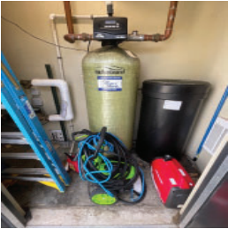
Gasoline stored inside, ladder blocking access to sprinkler system.
