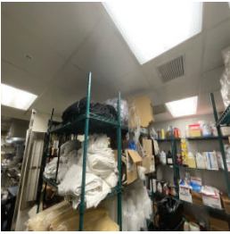
Storage too close to ceiling
