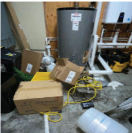
Storage in front of electrical panels
