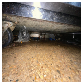
Wheels of appliance not in floor devices.
