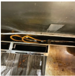
Cable restraint not attached.
