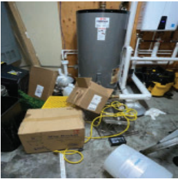
Combustibles in mechanical room
