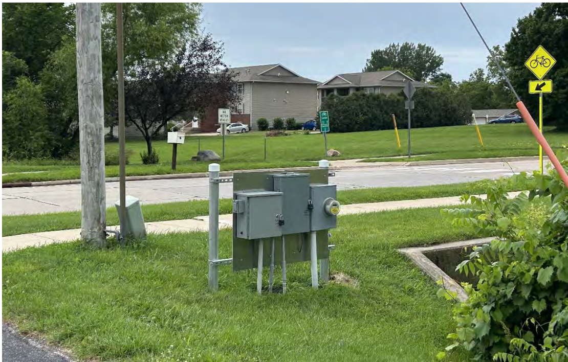
W Cherry St electric street light cabinet before and after
