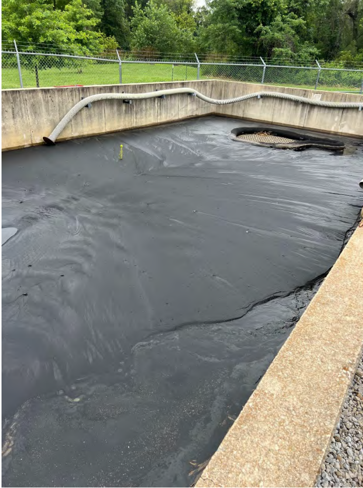
Sediment pumped from bottom of treatment tanks – Removed from system and hauled to landfill.
