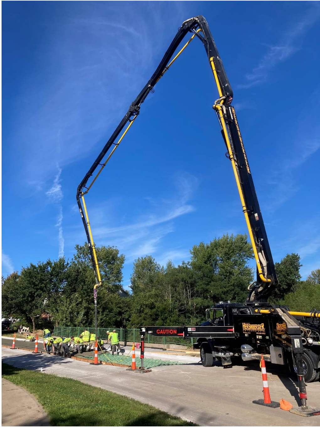
Rachael St north side repair. Staff using a pump truck in order to keep 1 lane open.
