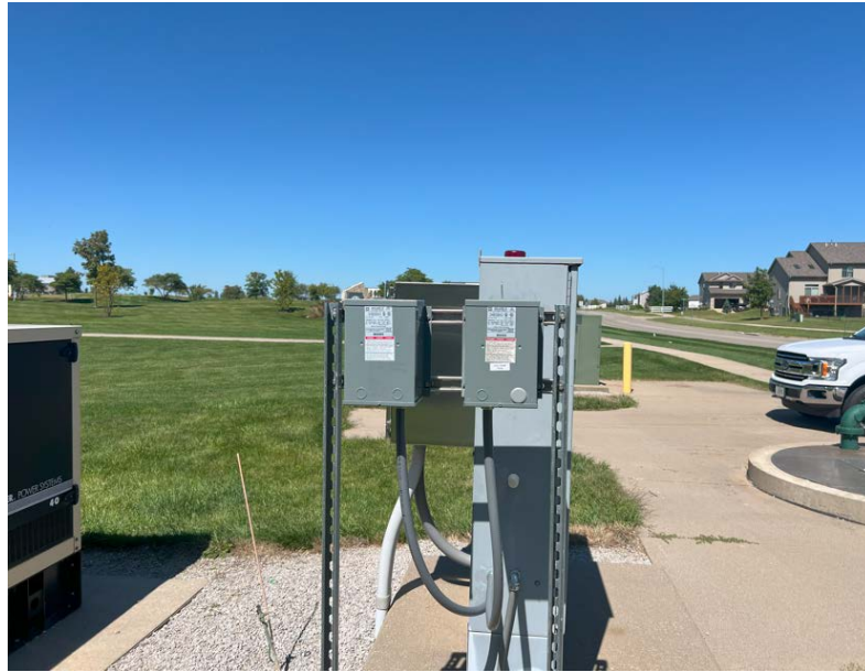
Re-located transformers at West Lake and Aspen Ridge Lift station.
