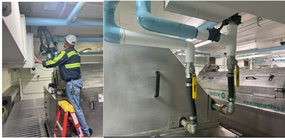
Replacement valves and pipe insulation on Parkson fine screen spray wash system.
