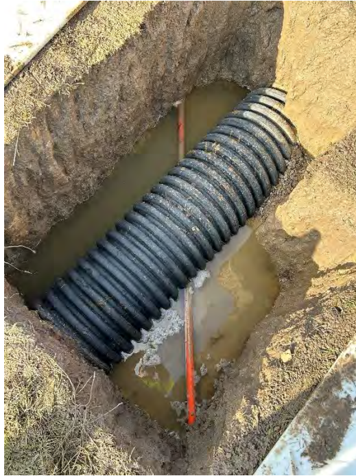
Storm pipe damaged by utility contractor
