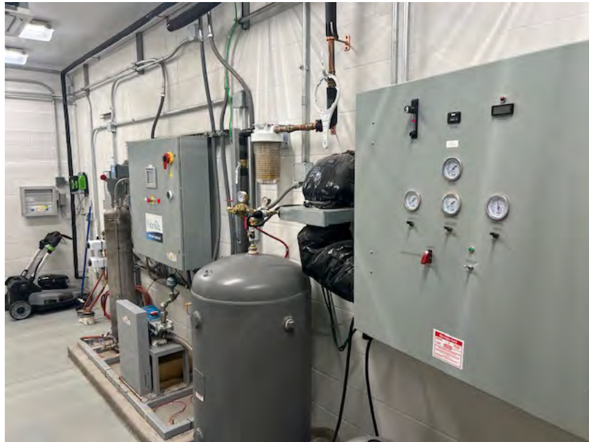
Complete Oxygen Generator System for H 2 S Treatment
